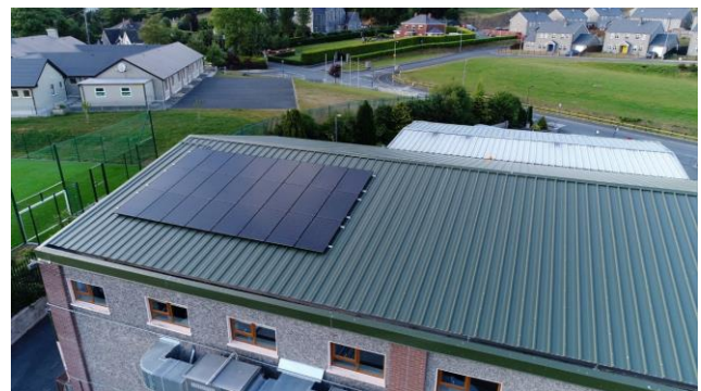
Corduff Raferagh Community Centre roof after upgrade works and installation of solar panels. Image credit: Corduff and Raferagh Community Association
