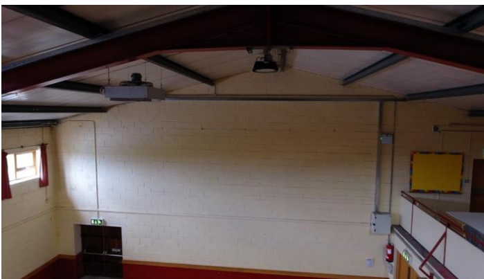
Ceiling of Corduff Raferagh Community Centre before upgrade works. Image credit: Corduff and Raferagh Community Association
