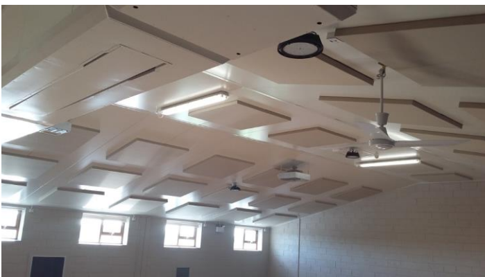
Ceiling of Corduff Raferagh Community Centre after upgrade works. Image credit: Corduff and Raferagh Community Association
